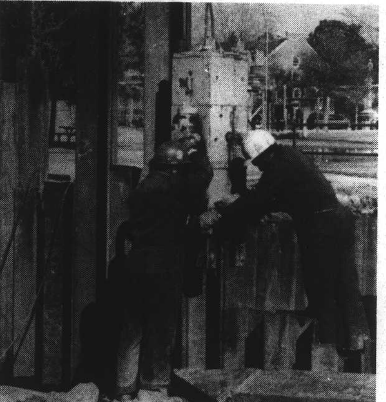
PARK BULKHEADING - Steel bulkheading is driven into place for the town's new park. The work is being done by Waff Brothers Construction Co., reportedly at an unusually good price.
