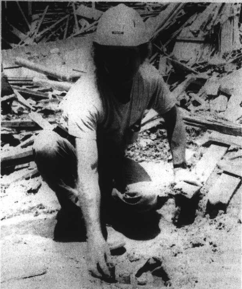
PROPANE -W.H. Weaver Co. foreman, Richard Winge holds the relief valve that was torn loose from a propane tank at the spot where the accident occurred. He is surrounded by debris that was being pushed into a pile by a bulldozer when its track severed the valve from the buried tank.
