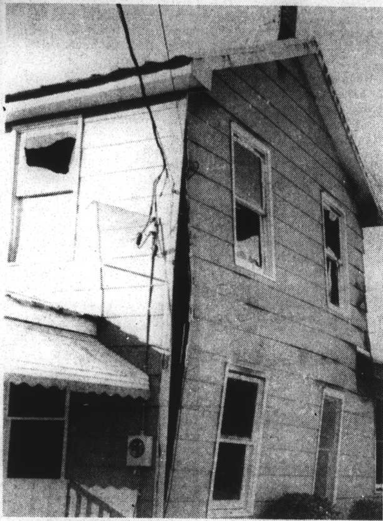
HOUSE BURNED --An arson investigation has begun by the Edenton Police Dept. and the SBI as the result of the fire at this house at 122 W. Hicks St. early Sunday morning. An explosion, believed to have resulted from use of an accelerant, bulged out the east wall. The interior was completely destroyed.
