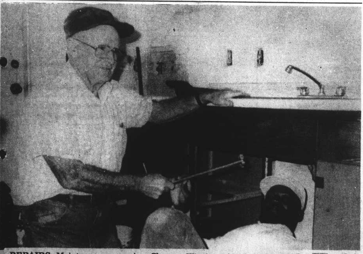
REPAIRS--Maintenance supervisor Clarence Wigginton hands a plumbing wrench to Jesse Moring as they prep an apartment for new tenants at the Edenton Housing Authority's Oakum Street site. Their maintenance shop is spotless with every tool in its designated place.
