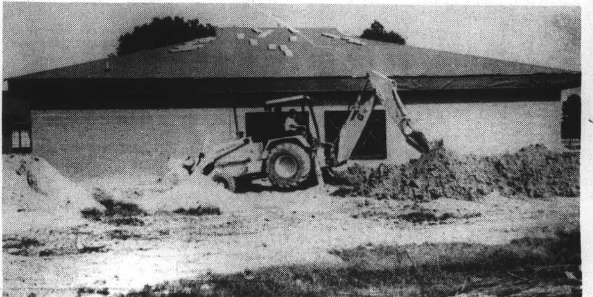
FINISHING UP-- The finishing touches were being put on the exterior of the new exceptional children's building at D.F. Walker last week. It is scheduled to be in use today for the first day of the school year.
