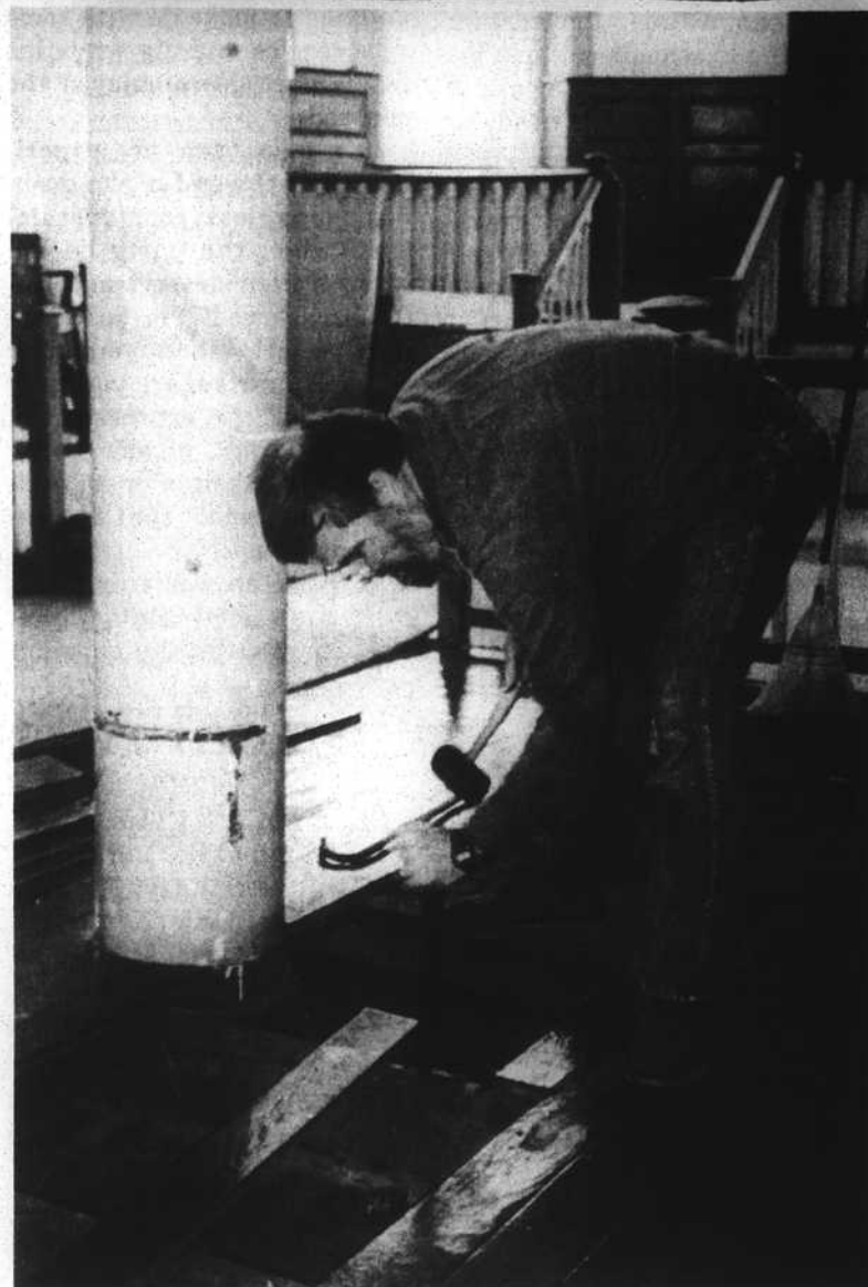
UNCOVERING THE PAST -- Don Jordan of Edenton removes flooring in the Old Chowan County Courthouse to reveal original stone paving beneath. The work is being carried out under the supervision of the N.C. Division of Archives and History and Colonial Williamsburg authorities, who will also conduct a study on this phase of the courthouse's revelations. An octagonal base supporting the column can be seen to the left of Jordan's hand. A section of the floor will remain uncovered for public interest and viewing. (Staff photo by Marguerite McCall.)
