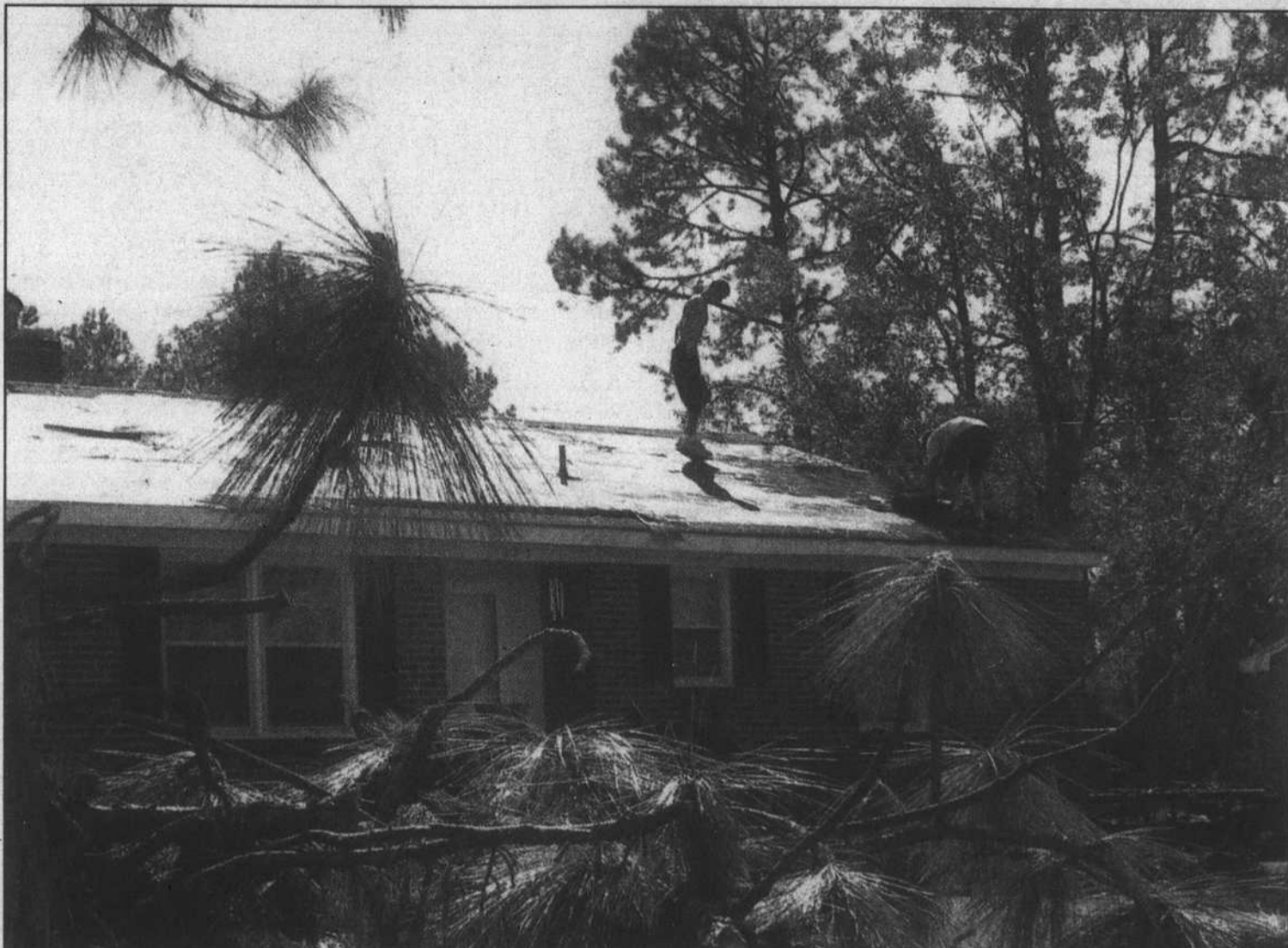
Repairing damaged roofs and water leaks are high priority jobs in Chowan County these days. Filled with "can do" spirit, local residents are taking the situation in stride and making strong progress toward cleaning up the debris left behind by Hurricane Isabel. Electricity, phone service and safe drinking water have now been restored to most local homes. (Staff photo by David Crawley)
