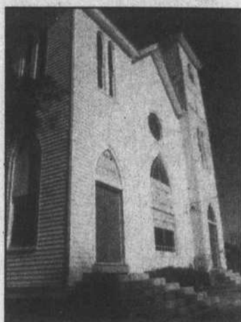
The historic Kadesh AME Zion Church in Edenton sustained heavy damage during Hurricane Isabel. Church officials estimate it could be years before all the damage is repaired. (Staff photo by Sean Jackson)
