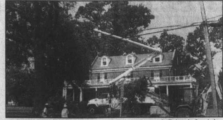
Town workers deal with a damage tree twisted in power lines on N. Broad St. Monday morning.
