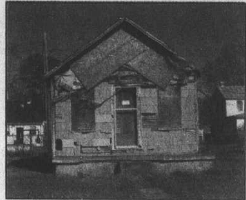
Vacant, run-down houses in Edenton are being considered nuisances by the town. They will either have to be repaired or demolished.
