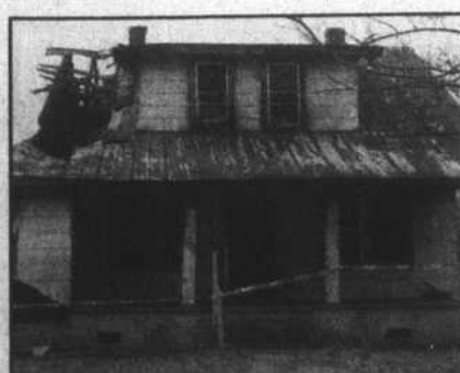
An abandoned house at 701 MLK was deemed a total loss after the fire.
