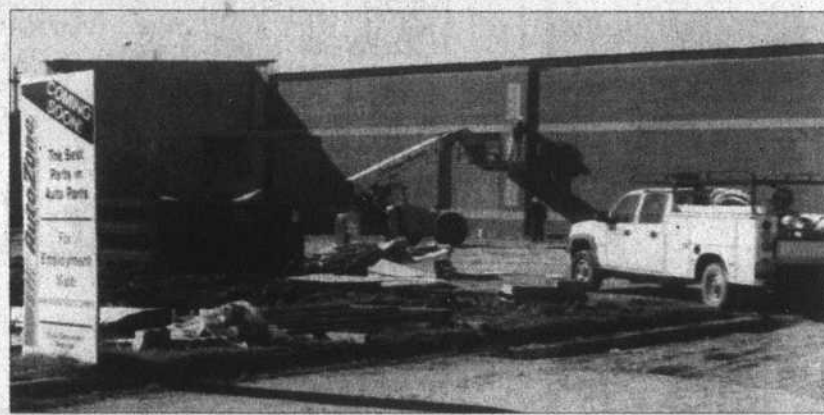
Workers finish up the construction of the AutoZone building on Virginia Road.
