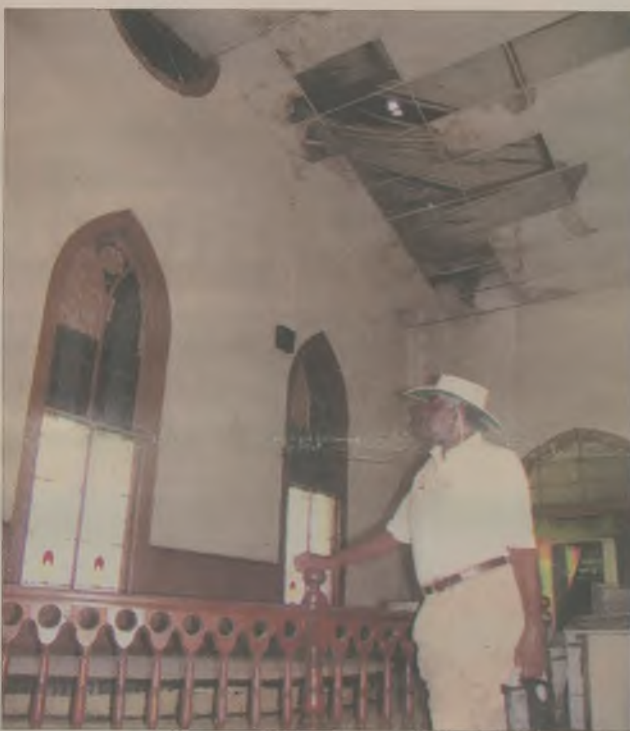
Kadesh A.M.E. Zion Church member Fred Joyner looks at boarded-up stained glass windows in the sanctuary following Hurricane Isabel. Above, the ceiling also shows damage from the hurricane's heavy rainfall.
