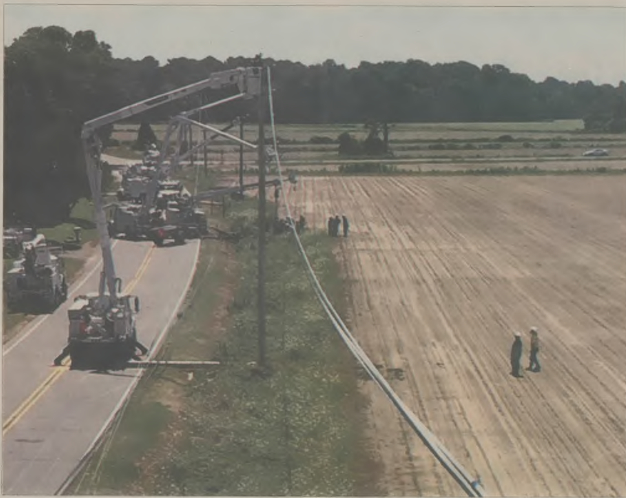
PHOTO BY ELECTRICITIES OF NC
