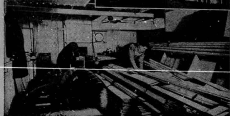
Elaborate alterations were made on the HMS Repulse to insure the finest possible quarters. The above picture was taken in early January when workmen began refitting the main dining room.
