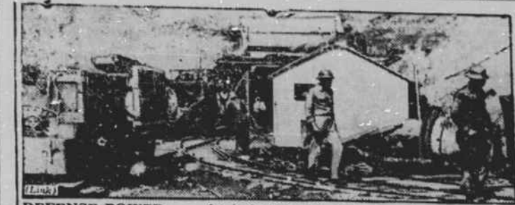
DEFENSE POWER . . . As industry and government sought more power to make aluminum for planes, work sped forward on Nantahala, N. C., dam, one of two hydro-electric projects building in southeast for Aluminum Company of America, already largest industrial customer of TVA and Bonneville. Part of firm's $150,000,000 defense expansion, project will have highest "head" east of Rockies.
