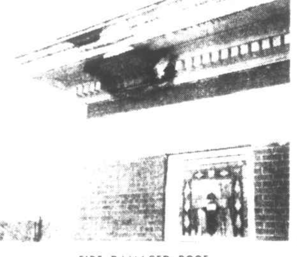
FIRE DAMAGED ROOF
