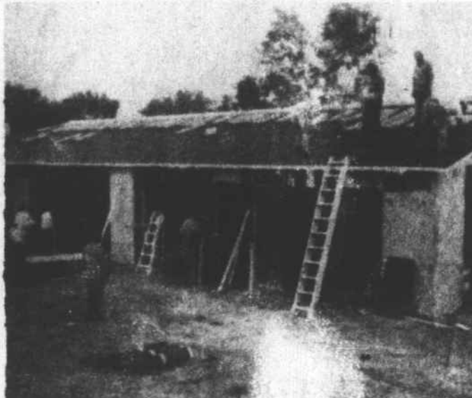
Here's a look at the sanctuary built on the Navajo Reservation before its completion. The project was paid
