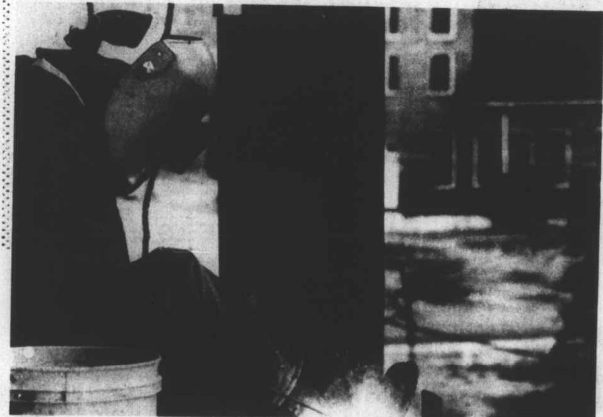
High above the hustle and bustle does some welding on the third floor of the PSU campus, Willie Locklear of the new addition to the Herbert G. Oxendine Science Building. [David Malcolm Photo]
