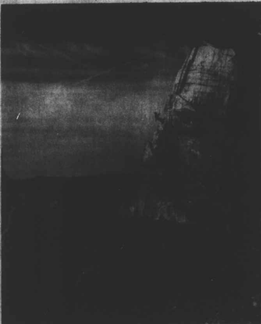
PROFILE EMERGING--With the recent removal of rock from in front of the chin, the full, nearly nine-story-high profile of Crazy Horse now is blocked out on the colossal mt. carving in progress in the Black Hills of S. D. (October, 1991 photo by Robb DeWall)
