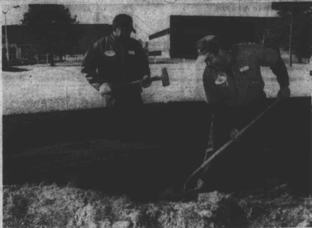
Archie V. Locklear (left) and William Michael Oxendine begin groundwork on Pembroke State University's new main entrance, which is to be located off Odum Road, in front of the University's new administration building, seen at left in the background. (PSU photo by Bobby Ayers)
