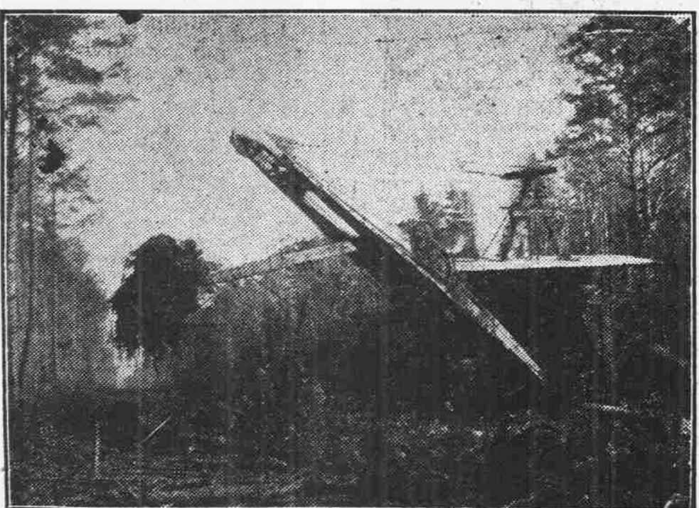
THE type of steam dredge commonly used in cutting canals in drainage districts in Eastern North Carolina.
