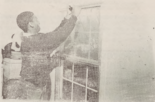
Installing Storm Window — Harry Harvin, a weatherization assistant, with the Energy Office of Operation Breakthrough, installs a storm window in a home the agency recently weatherized.
