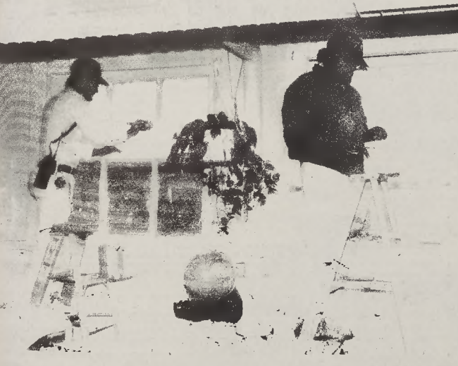
WORKMEN correcting the problem of lead at Operation Breakthrough. (Photo by Ray Trent)
