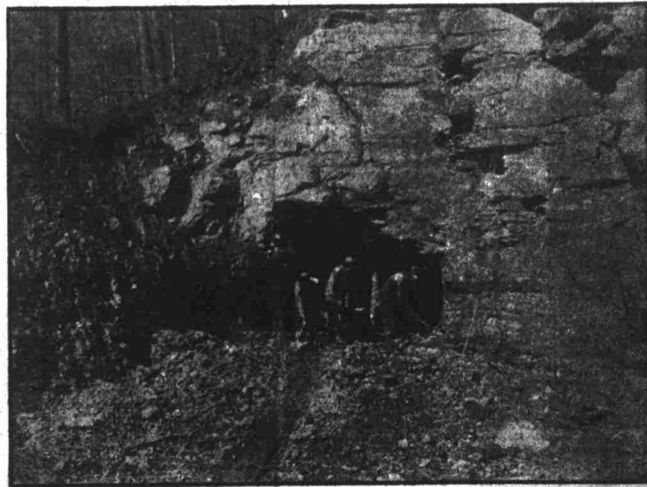
Making a "Clinchfield" entry, preparatory to beginning the removal of coal by the train load.
