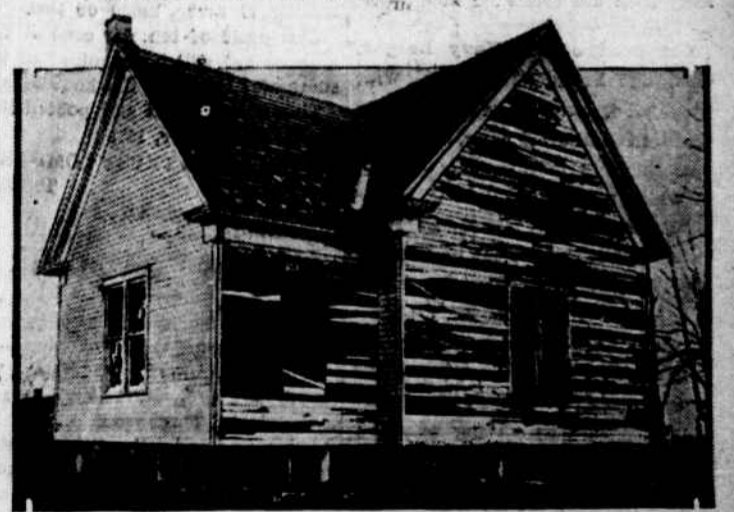
THIS is the Methodist church at Rayville, Mo., after hailstones as large as baseballs and blown by a 60 mile gale had demolished the sides of buildings which were exposed directly to the wind. Weather boarding was smashed, windows broken and shingles torn off.
