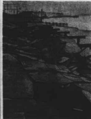
This picture, taken on the ocean front at Redondo Beach, Calif., shows how tides and pounding waves have turned the concrete walkway into a series of broken blocks.
