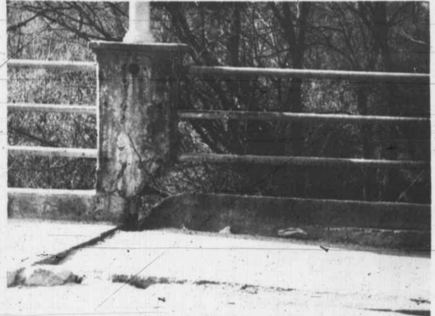
Bridge In Poor Repair
