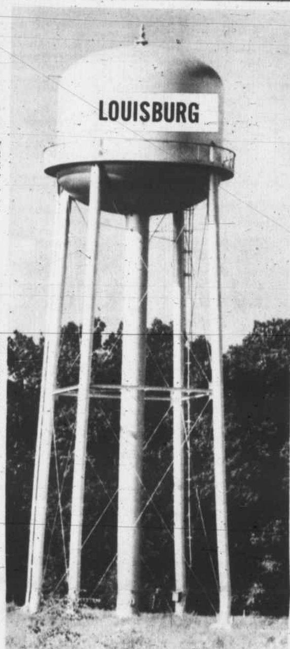
Water Storage Tank
