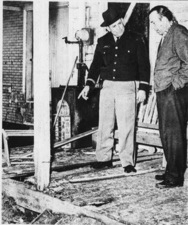
Deputy Sheriff Lloyd Gupton Views Dynamite Damage With Store Owner Jack Collins.
