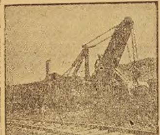
(These machines lift five tons or more at once, and can load a car in three minutes.)
