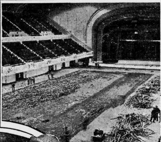
WPA WORKING FOR G.O.P.—Carpenters for WPA building a new floor in Cleveland's Public Auditorium. Two shifts are being used to complete the job in time for the Republican Convention to be held June 9.
