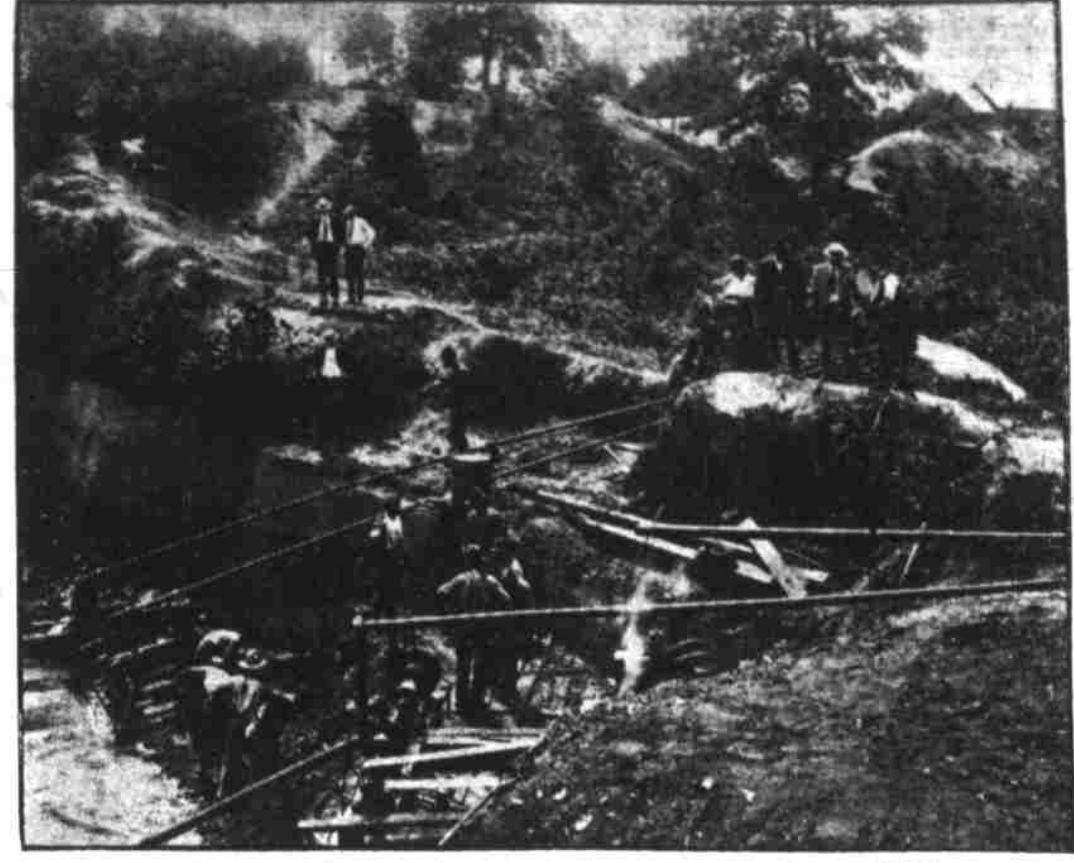
The two pumps in the center of the picture ran 28 hours without a stop, or from 2 o'clock Saturday afternoon until 6 o'clock yesterday afternoon when the power was shut off so they could be moved down into the quarry. Over at the left one of the State's Community Service men is taking some moving pictures that will later be shown in funds of school houses throughout the commonwealth. The very interested spectator looking at the camera is not Fatty Arbuckle, but Captain Christian, superintendent of the Prison Farm. Behind the movie camera can be seen the stream of water thrown out by the two small pumps.
