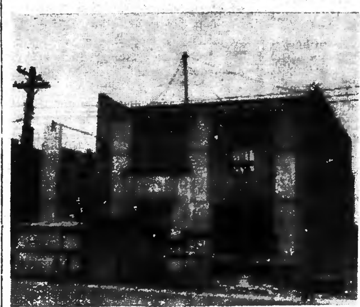
Here is pictured North Wilkesboro's city hall under construction. The building, which will house all departments of the city government, is being erected as a Public Works administration project at a cost of approximately $33,000. It will be ready for occupancy within a few weeks.
