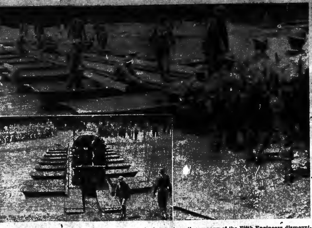
In a demonstration at Ft. Belvoir, Va., a motorized war-strength company of the Fifth Engineers dismantled from its trucks, unloaded equipment, and within 16 minutes constructed a 200-foot pontoon bridge strong enough to carry ammunition trucks. In picture at right, runways are laid across gunnels of light pontoons. Inset: Company "E" of the Fifth Engineers is shown crossing waterway on bridge.
