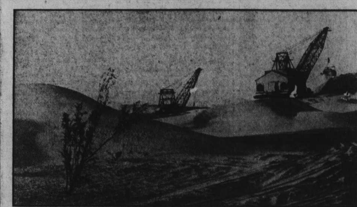
Moving huge barriers of ever-shifting sand, these powerful draglines, operated in 24-hour shifts, are excavating for the All-American canal across the southern California desert country. The canal eventually will carry water from Boulder Dam into the Imperial Valley.
