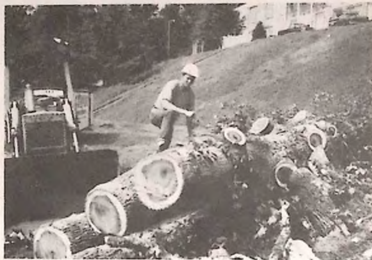
Drew Sheppard of Cooper Construction atop the large poplar tulip tree that was felled to make way for the new Saluda School Buildings recently. (Photo by Ceri Dando) —Community Reporter
