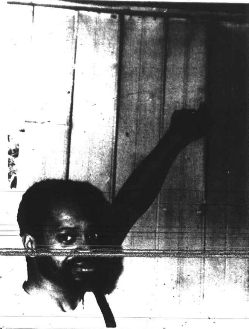
An angry resident of the Liberty-Patterson area demonstrates a crack in his ceiling.
