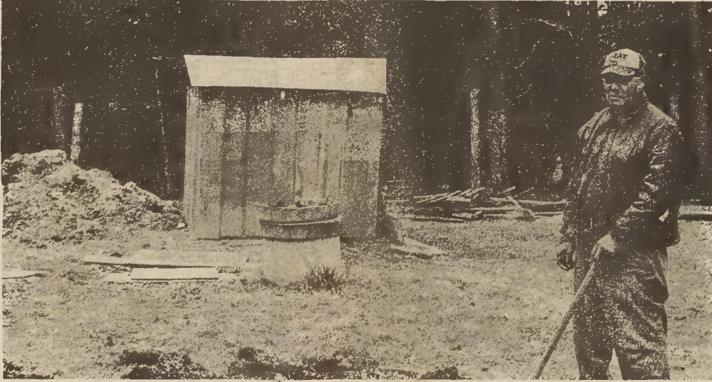
Wade O'Neal of Grove Garden Road is in the process of digging a trench to lay pipes, so he can be reconnected to city water. O'Neal and his family have been without water since November.
