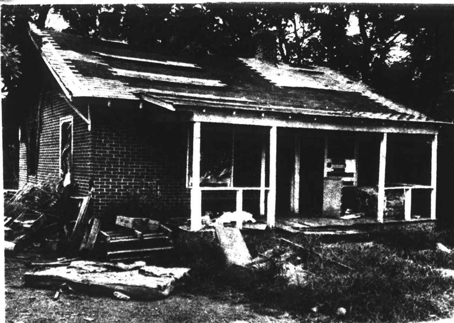
An abandoned house that has been deemed unsafe by city inspectors (photo by James Parker).
