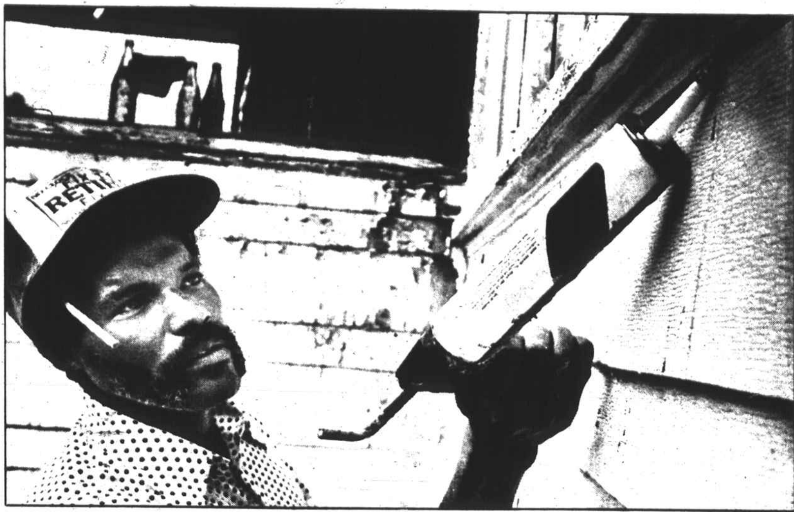
Calvin McDaniel Jr. caulks around the window of a Patterson Avenue home (photo by James Parker).
