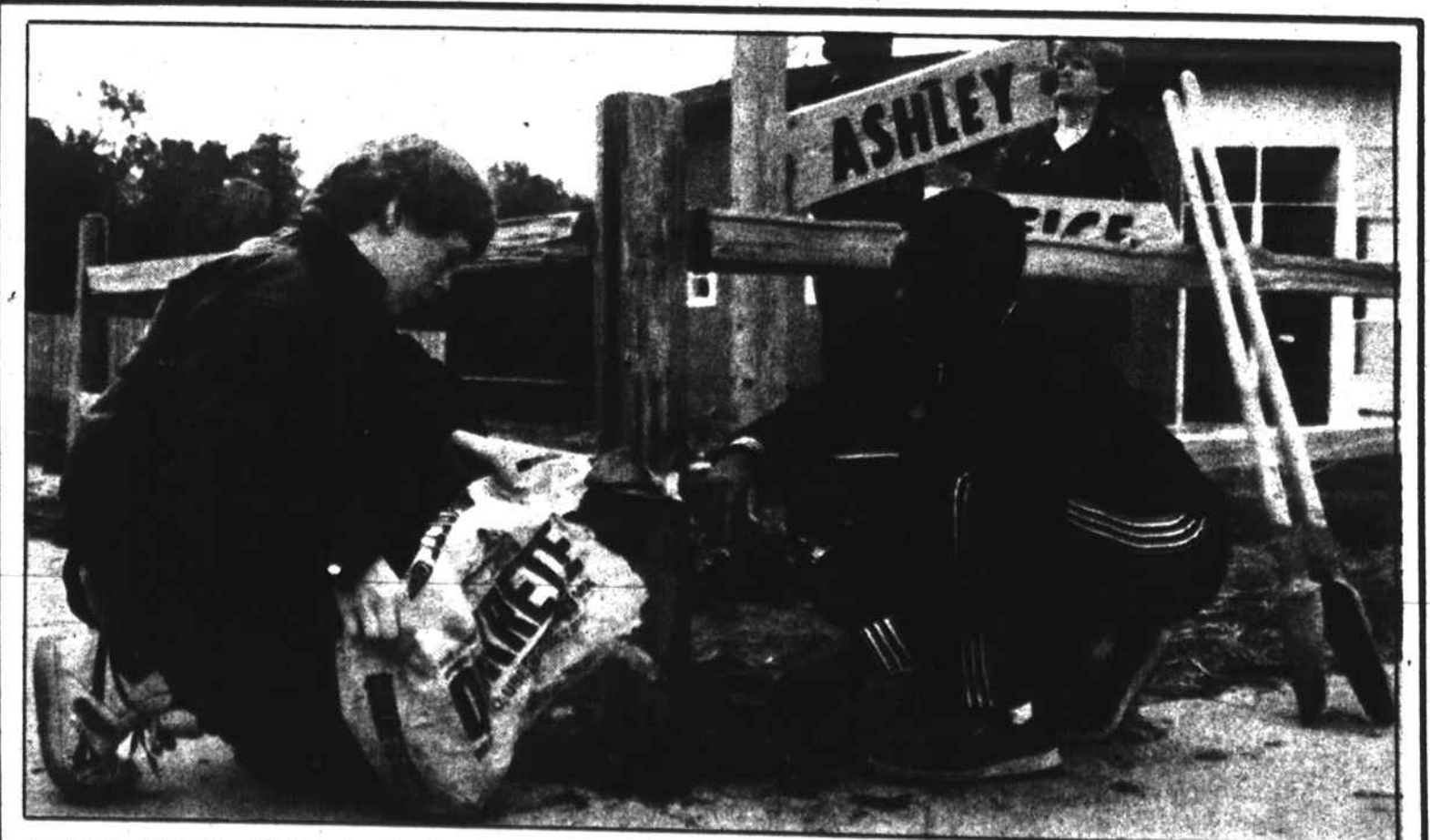
Ashley Middle School students work to replace the fence that was torn down by vandals (photo by James Parker).
