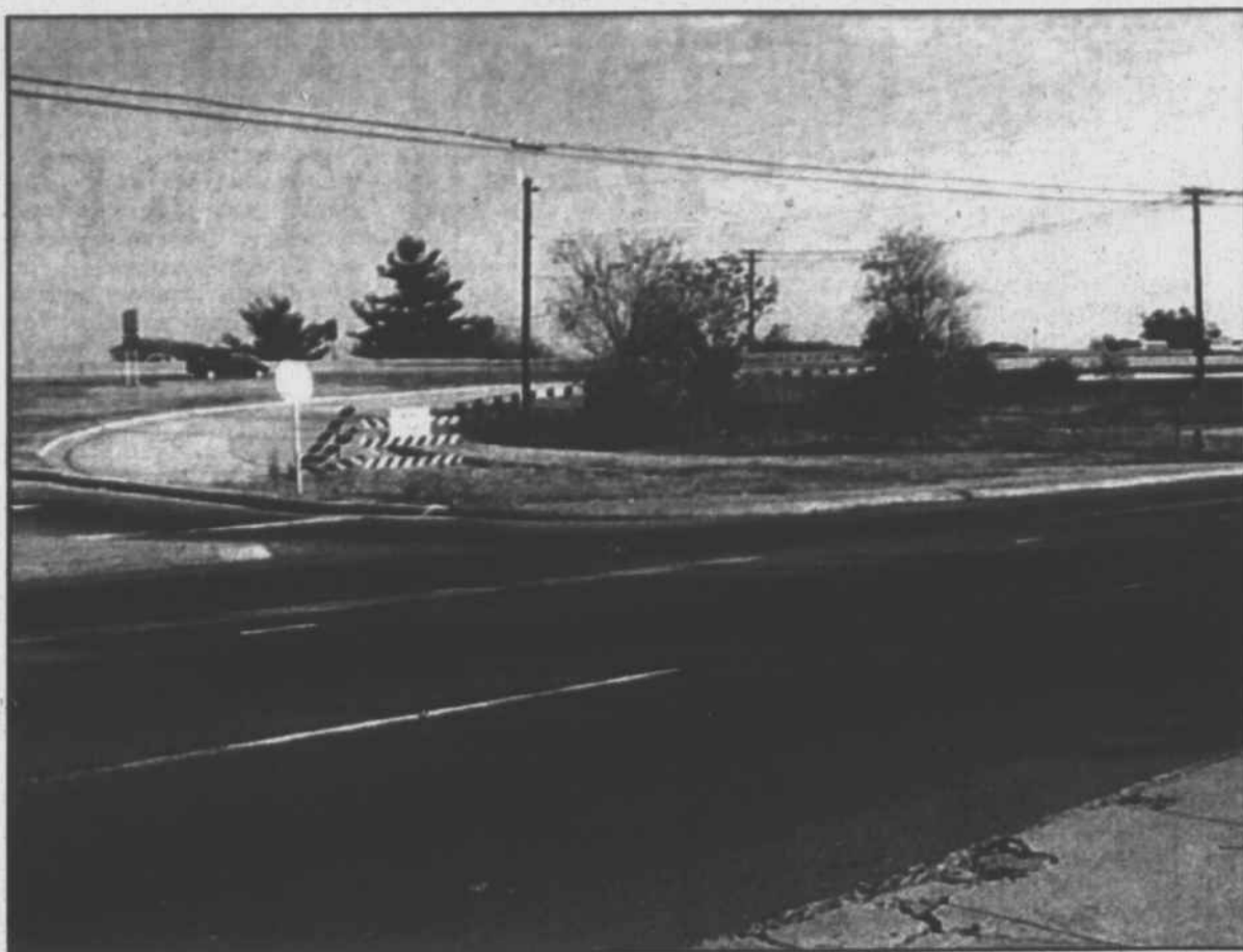
Photo by Bruce Chapman An exit from Liberty Street to US-52 is still incomplete. Plans to convert the highway into I-74 could bring improvements to the area.
