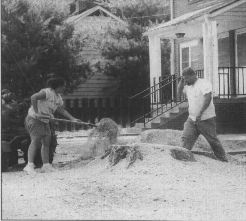
Workers prepare the area where trees were cut down in Cleveland Avenue Homes.
