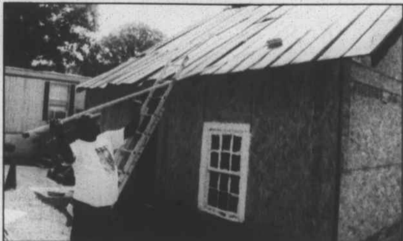
Photo by Todd Luck Carpenter John Robertson paints the roof on a farmhouse built 110 years ago by a former slave. To read about the effort to restore the house, see page A2.
