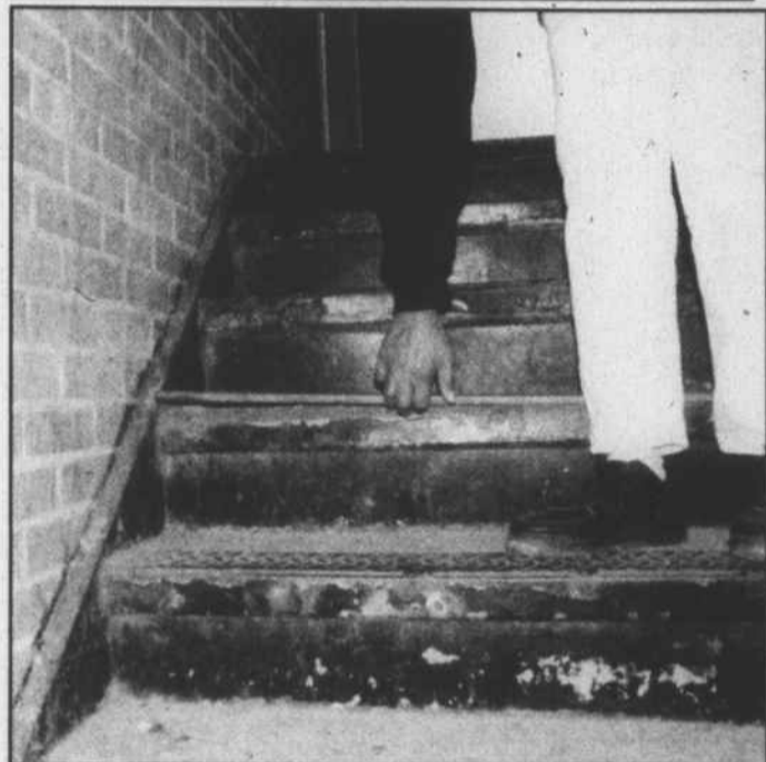
A picture taken in a Rolling Hills stairwell in 2009 shows some of the structure's wear and tear.
