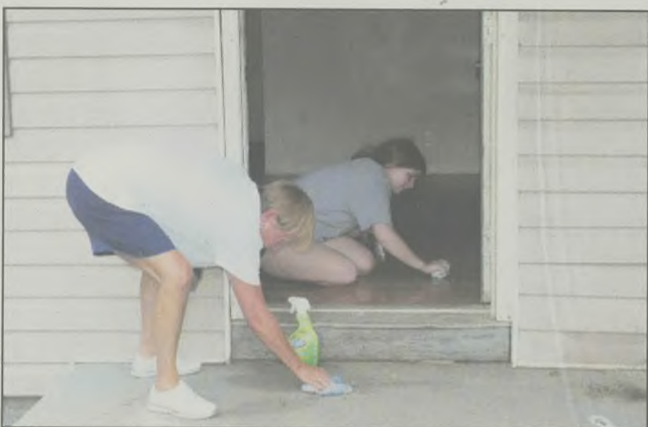
Volunteers have put in countless hours of work to make sure they make their end-of-August deadline for the renovations.
