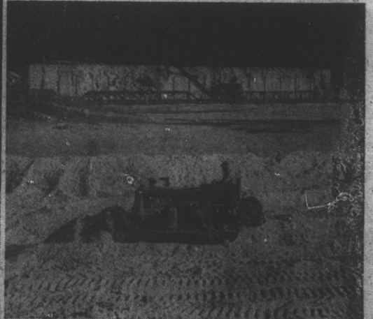
Bulldozer works on storage vat where molten sulphur can cool and harden like huge block of sulphur in background.
