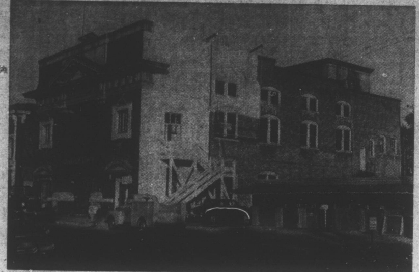
CITY HALL GETS FACE-LIFTING — At long last—and long past due—Dunn's old city hall is getting a little touching up. City policemen and other town employees were used to paint the interior. It looks like the building is being painted, but City Manager Oliver Manning says it isn't paint at all, but is being waterproofed with a special preservative known as Stadri. It fills up all the holes and cracks and completely waterproofs a building. The building has to be sprayed with water and thoroughly wet before application is made. Anyway, it has the same appearance as paint and is a big improvement. Joe and Cyrus Goodman are doing the job. (Daily Record photo by T. M. Stewart.)
