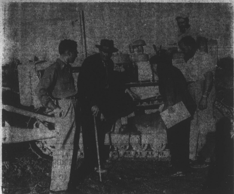
WORK BEGINS ON NEW HOUSING PROJECT — C. T. Latimer, president of C. A. Latimer, Inc. is pictured here with City Manager Oliver O. Manning and construction men as work got underway Friday on a new $200,000 housing project to be known as Woodlawn Subsection No. III. Twenty-two modern new homes will be built for resale and the project is due for completion by April 1. The big bulldozer is one of many fine pieces of grading and excavating equipment owned by Lewis Godwin Co., local grading contractor. Left to right are: Derwood Godwin, Mr. Latimer, City Manager Manning and Mr. Godwin. The bulldozer operator was not identified. The new development is located on the Dunn-Erwin highway, just west of the Cumberland Street intersection. Mr. Latimer has already completed more than 100 homes in that section. (Daily Record photo by J. W. Temple Jr.)
